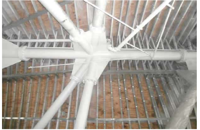
Interior Picture of Box Beams Spanning Between Circular Tube for Support. Photo courtesy of ADTEK Engineers, Inc.
