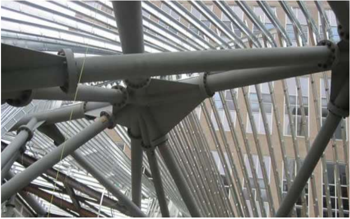
Interior Picture of Curved Stud Profile and Roof Looking Up. Photo courtesy of ADTEK Engineers, Inc.
