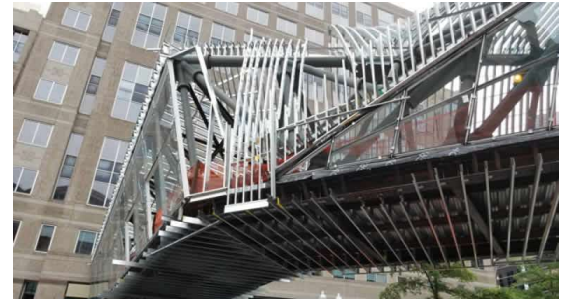
Exterior Picture of Curved Stud Profile and Soffit Framing Underneath the Bridge. Photo courtesy of ADTEK Engineers, Inc.
