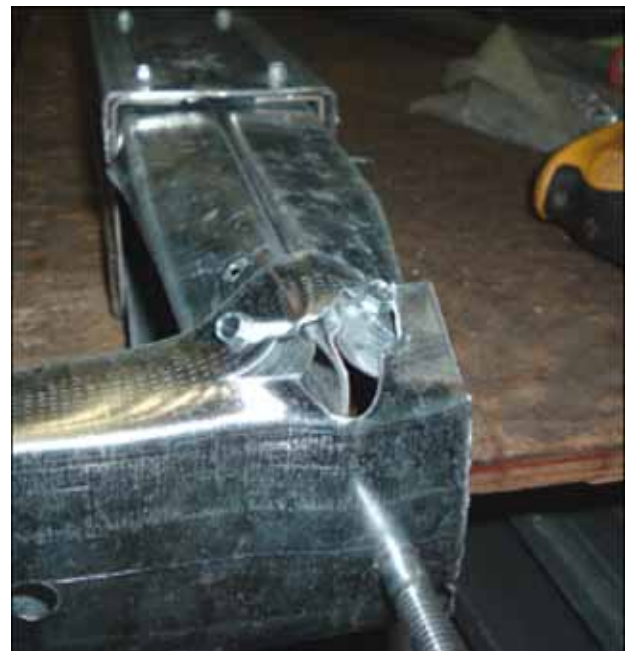
Figure 4: Punch-through failure at end of track.
