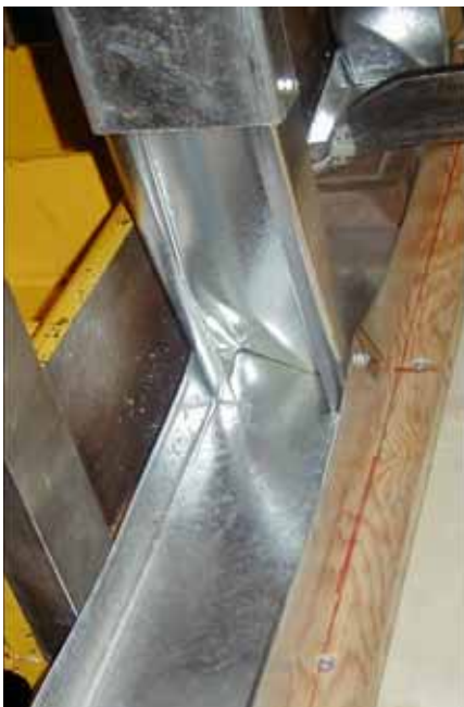
Figure 3: Single stud failure in track.
