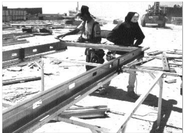
The ideal table for component framing is waist-high, quick and easy to adjust, and can be easily transported to and set up at the job site.
