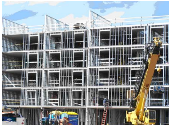
The six story Hilton Garden Inn, Durham, NC, pictured in February, provides an example of a structure built with cold-formed steel load bearing walls and precast hollowcore slabs.
